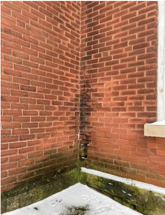
Plate 31: Location of former downspout on east elevation
